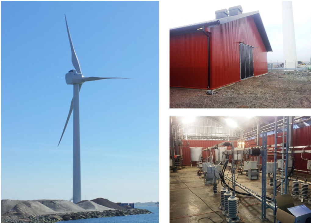
Figure 3. Testing facility in Gothenburg comprising the 4.2 MW FPC “Big Glenn” wind turbine; housing of the back-to-back HVDC station, and coupling inductor (back) and AC filters (front) inside the house.
