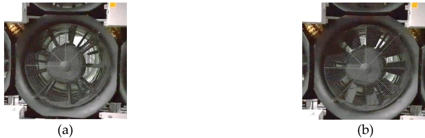
Figure 3. The adjustable vanes at the inlets of the 60 fans wall, (a) 100% open vanes, (b) 70% open vanes
