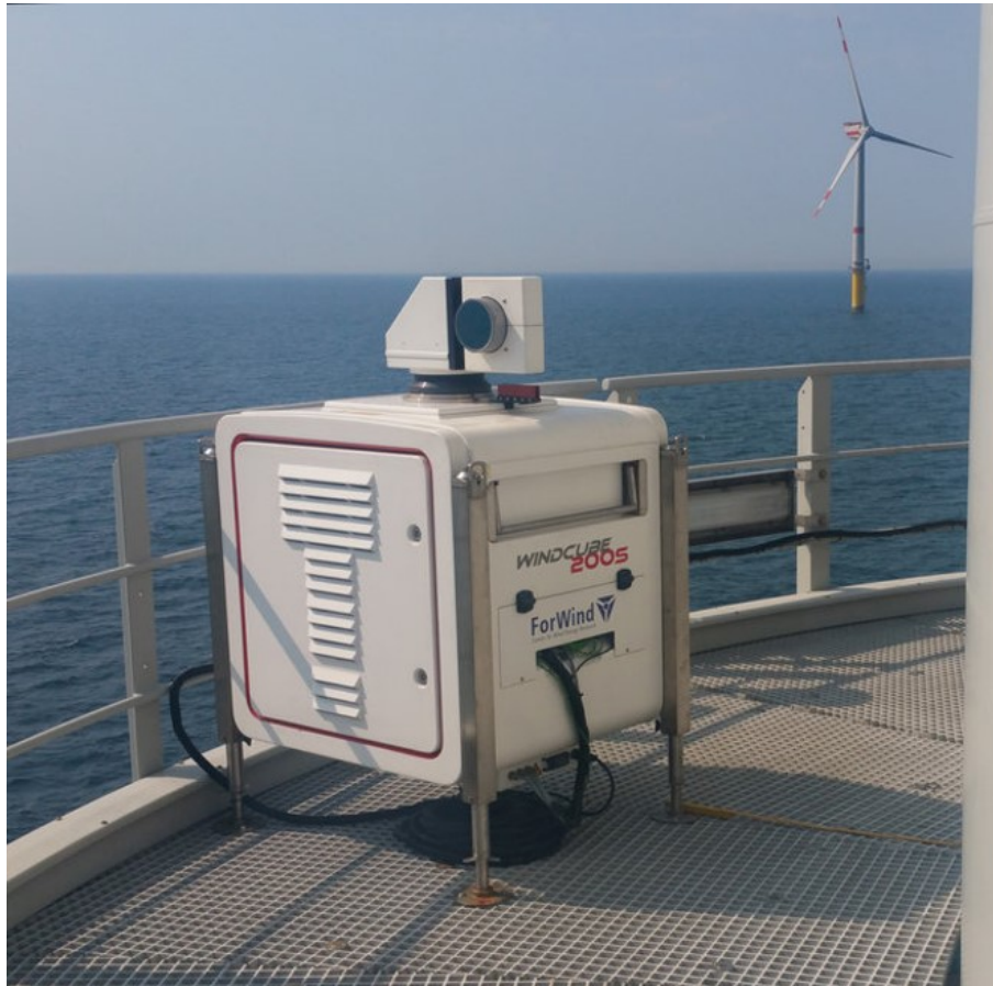
Figure 7. Image of the WindCube200S installed on the transition piece of the wind turbine in the offshore windfarm Global Tech I. Picture taken by Stephan Voß.
