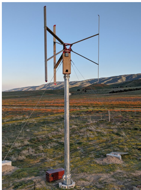
Figure 9. XFlow’s 5-kW prototype VAWT at the Field Laboratory for Optimized Wind Energy in Lancaster, California.
