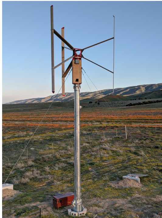
Figure 8. Photo of XFlow’s 5-kW prototype VAWT at the Field Laboratory for Optimized Wind Energy in Lancaster, CA
