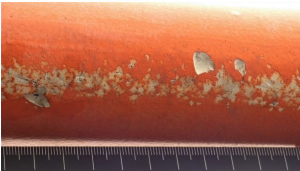
Figure 18. LEE damage on the tip section of a WTB, photographed by TNO
