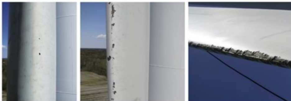
Figure 18. Changes to the LE surface due to impact with a different degree of severity, From left: LEE at an early stage, severely damaged coating and LEE starts to wear the shell material. Adapted from Keegan et al. (2013); Rempel (2012)
