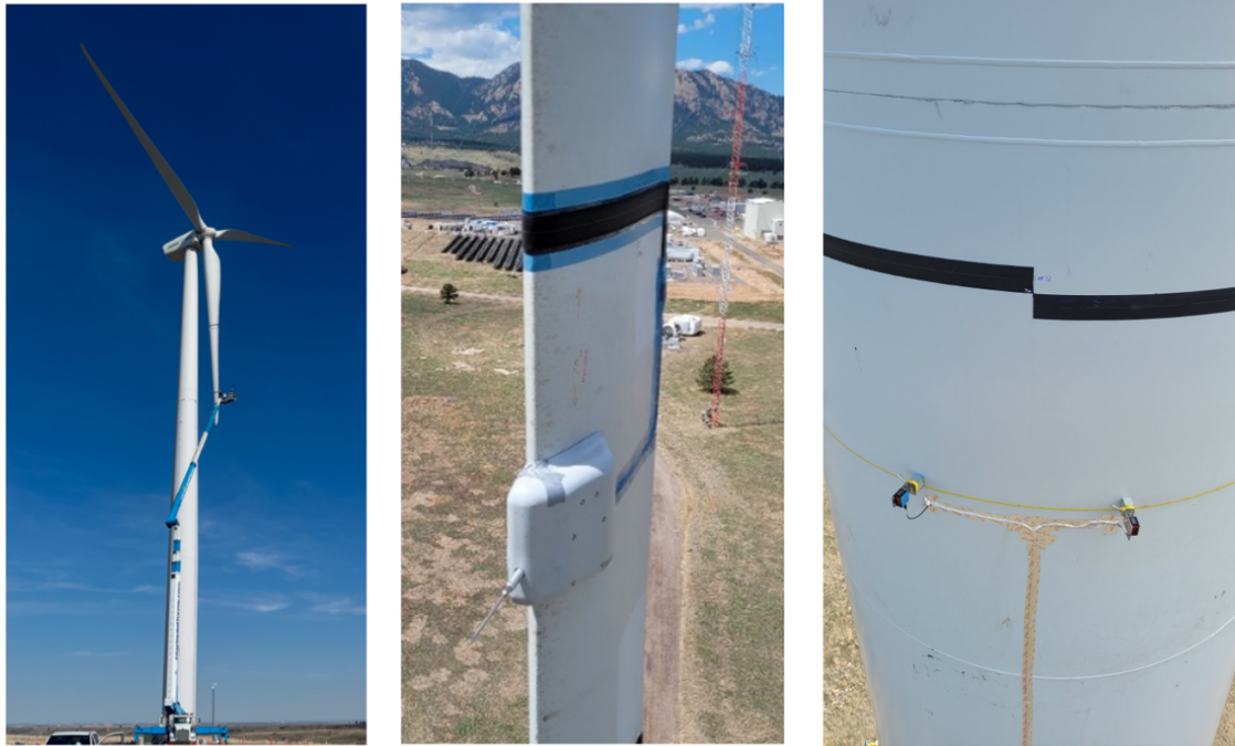
Figure 9. (left) Installation of the outer belt on blade 1 of the GE 1.5 MW wind turbine. The rotor is parked in a downwind configuration. The inner belt and flyboard are visible at the mid-span of blade 1. The belt on the tower had not yet been installed when this photo was taken. Photo credit: Pietro Bortolotti, NREL. (middle) Close-up view of the flyboard, five-hole probe, and belt installed at the outer blade location. Photo credit: Per Hansen, DTU. (right) The belts on the tower, each covering half of the circumference, were installed 1 m above the laser sensors and at the height of the outer belt on blade 1. Photo credit: Per Hansen, DTU.
