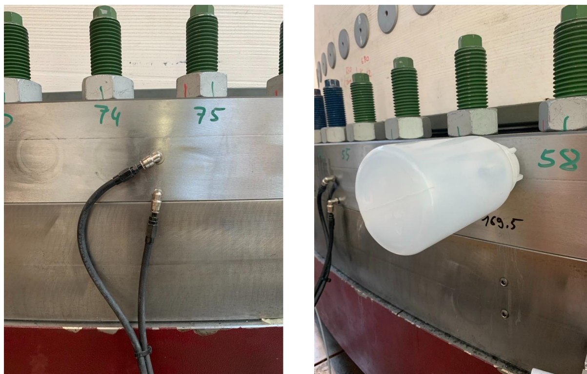
Figure 2: Grease inlets and outlets on the outer ring of the lower bearing
